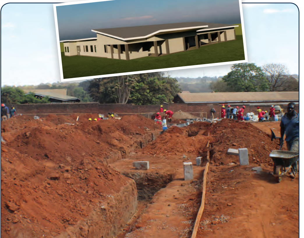
New STI clinic construction starts at Bwaila: A generous gift from Hyman and Marietta Bielsky will fund a new clinic at Bwaila Hospital, Malawi for reproductive health and sexually transmitted infections. The new clinic will replace infrastructure some of which constructed in the 1950s and has recently been used for sexually transmitted disease research and care. Photo: Innocent Mofolo
